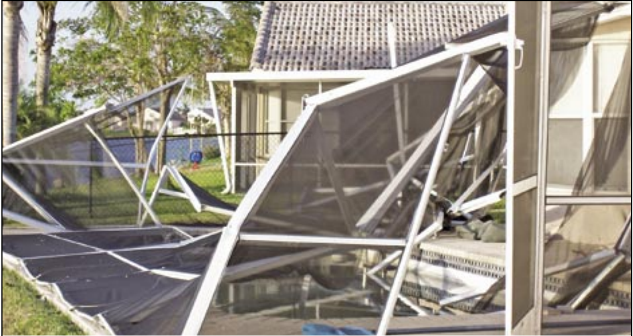
Due to last year's active hurricane season, many pool screens have been damaged and enclosure builders are more than a year behind schedule.
