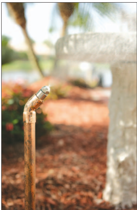
SWAT Mosquito Systems installs a custom-built misting system which releases a fine mist through a series of stainless steel and nickel-plated nozzles.
