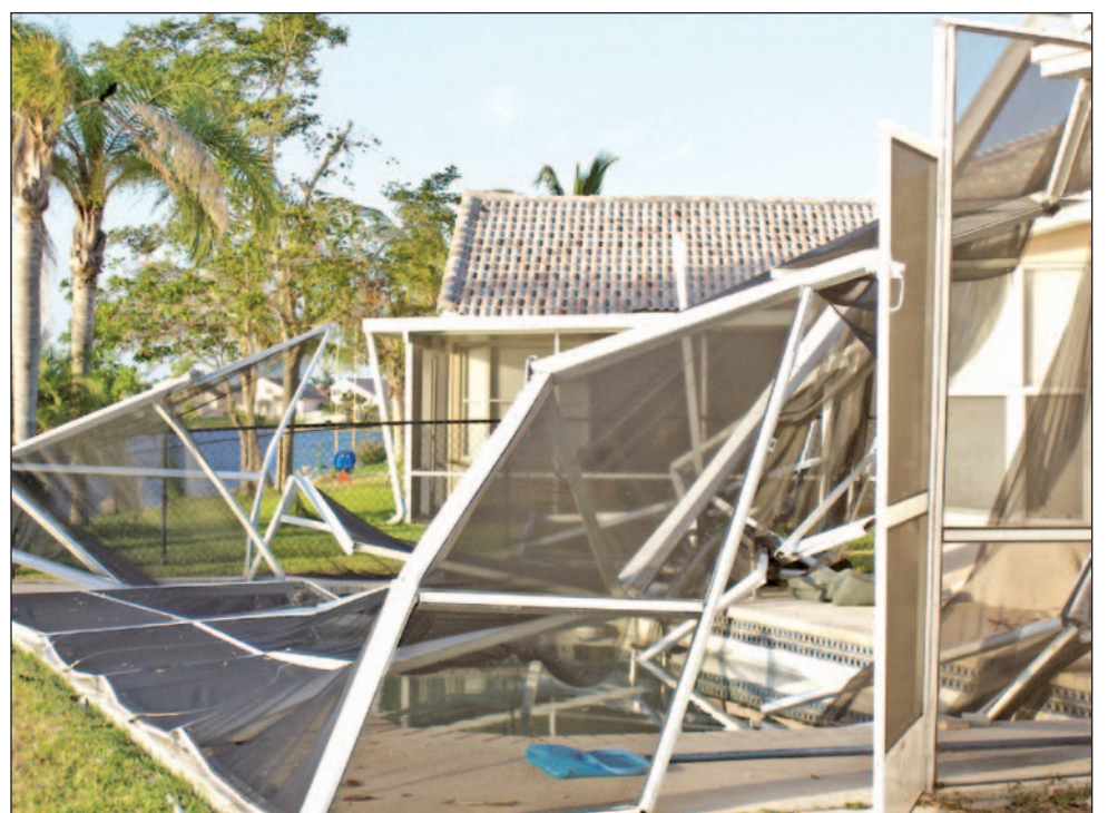
Pool screens took quite a beating during last year's storms forcing homeowners to wait more than a year for repairs.
